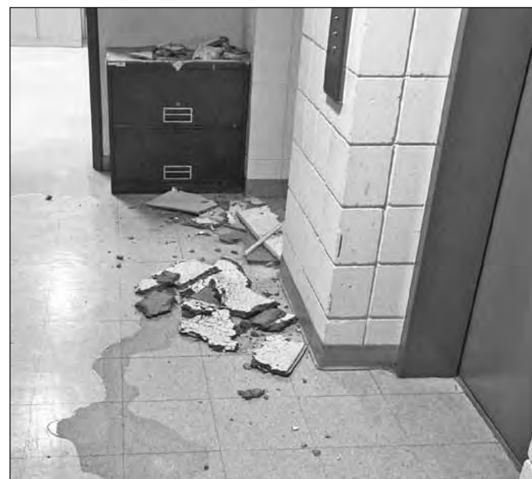
Ceiling damage at York College.
